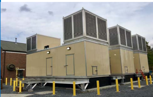
The new 1250 KW diesel Generators now in operation at the Authority Complex .
